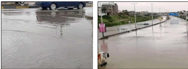
Fig. 8: Accumulation of water on asphalt roads
