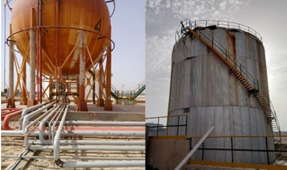
Fig. 4: Shows of tanks corrosion.
