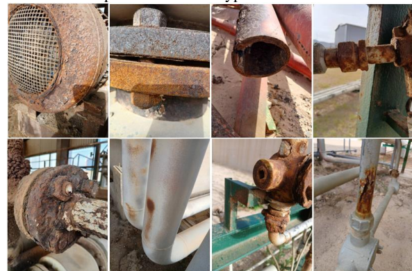
Fig. 2: Some types of corrosion.
