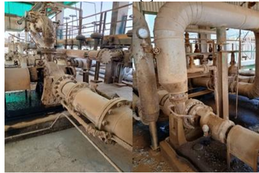
Fig. 5: Some failure parts caused by corrosion.
