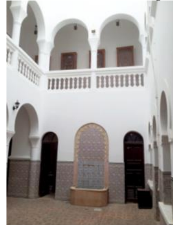
Fig (4) Columns and arches as structural elements to support the building. (The previous reference p.5)
