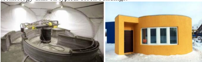
Fig. 12: The first on-site 3D printed house in just 24 hours in Russia by Apis Cor [37]
